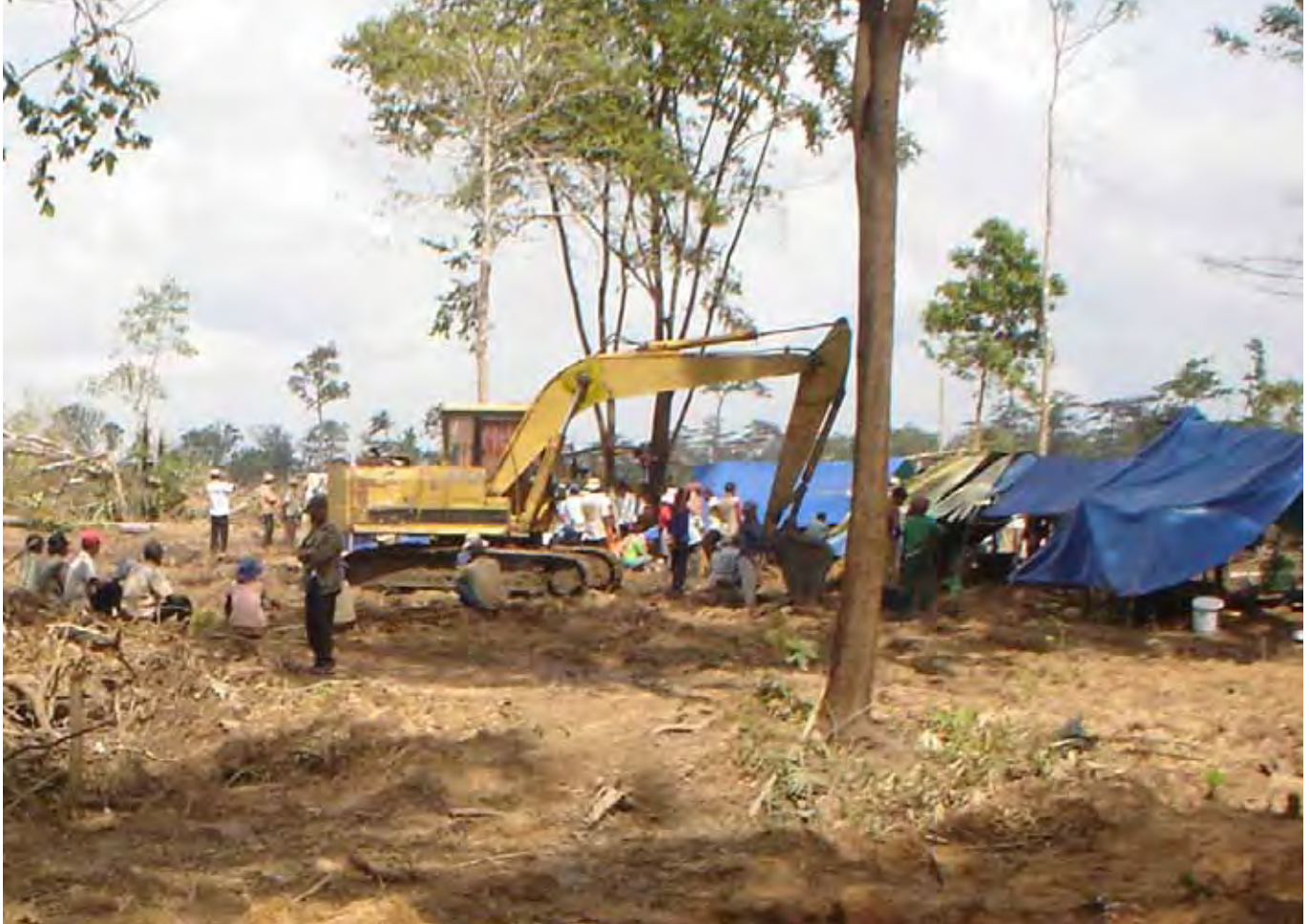
Village residents were surprised in July 2008 when they found their farmland in Snoul district was being cleared for a rubber plantation they knew nothing about. They protested and company workers dismantled the site. The case is now at the provincial criminal court.
