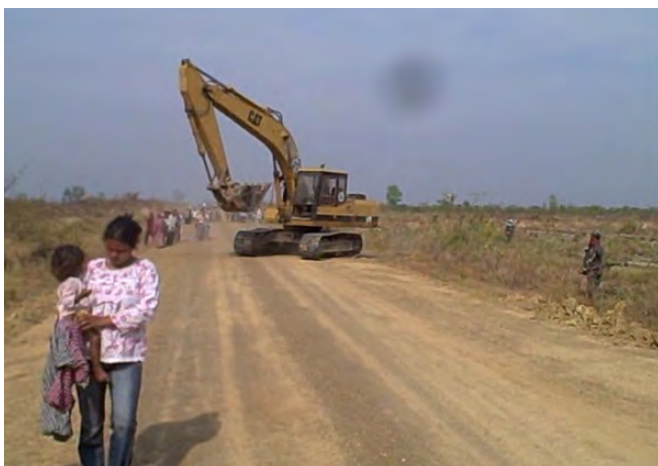
An excavator operating for CIV Company cleared a boundary ditch in an area previously agreed to remain as community land. CIV Company said it will still take 970 hectares of land.
